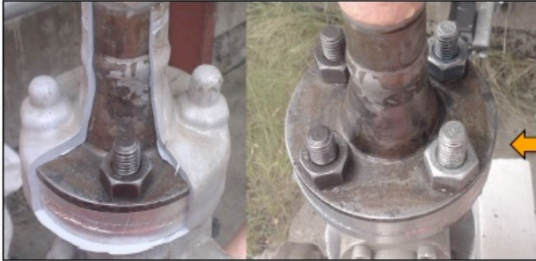
Flange coating removed by client after 1yr - No corrosion
